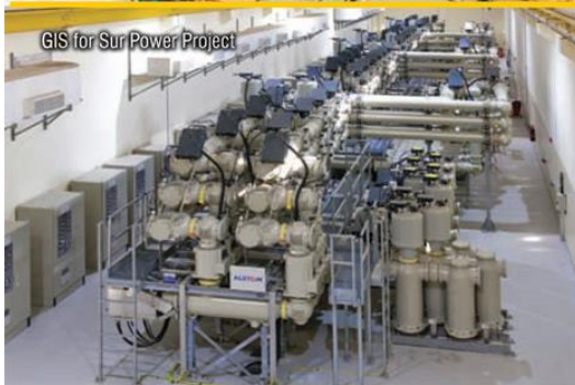
Sur Independent Power Project
